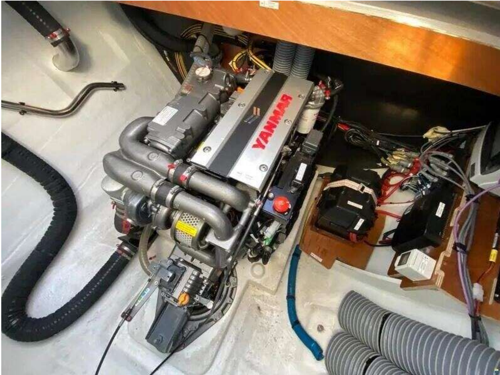
Engine compartment: Yanmar 4JH80 saildrive, batteries and service runs
